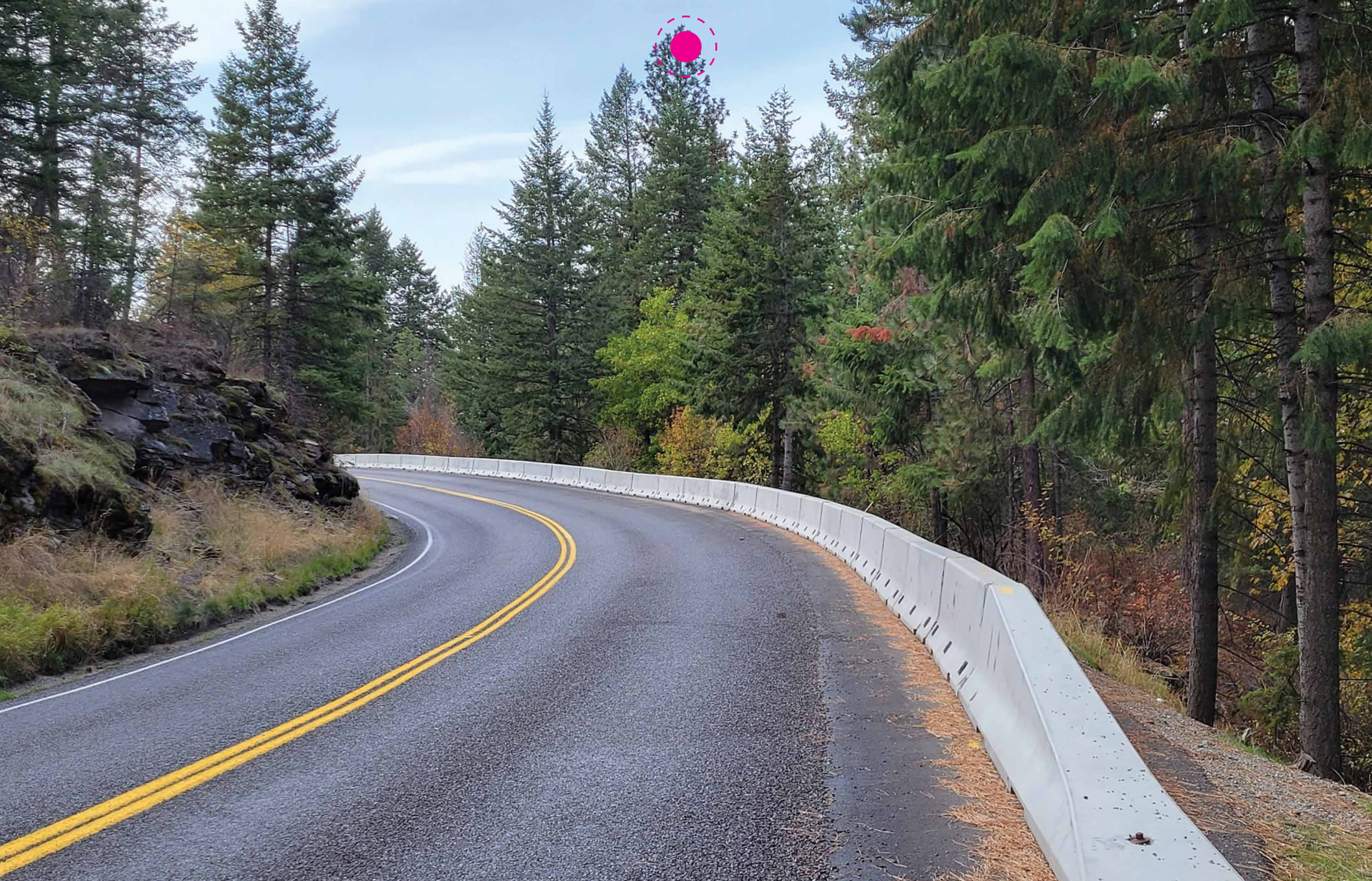
Rebecca Howell, LHTAC New Guardrail on Riverview Drive Post Falls Highway District
